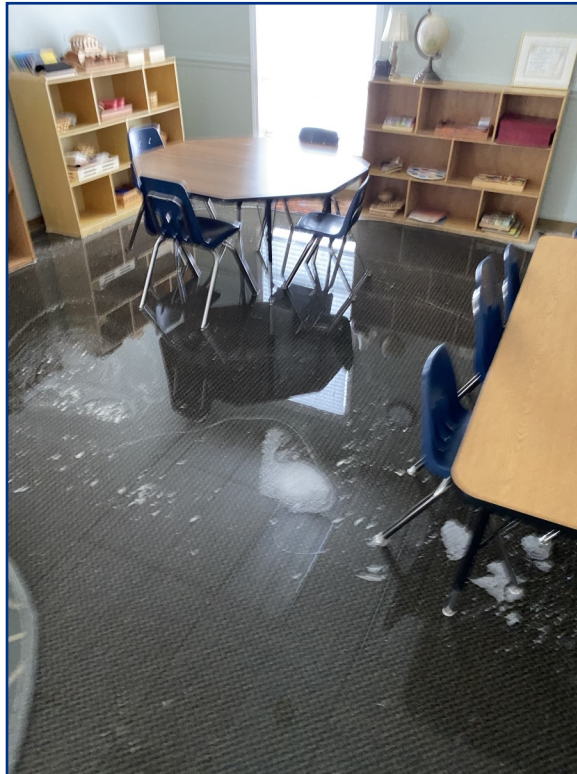
Water poured from burst pipes, flooding our children's wing and offices on December 26.
